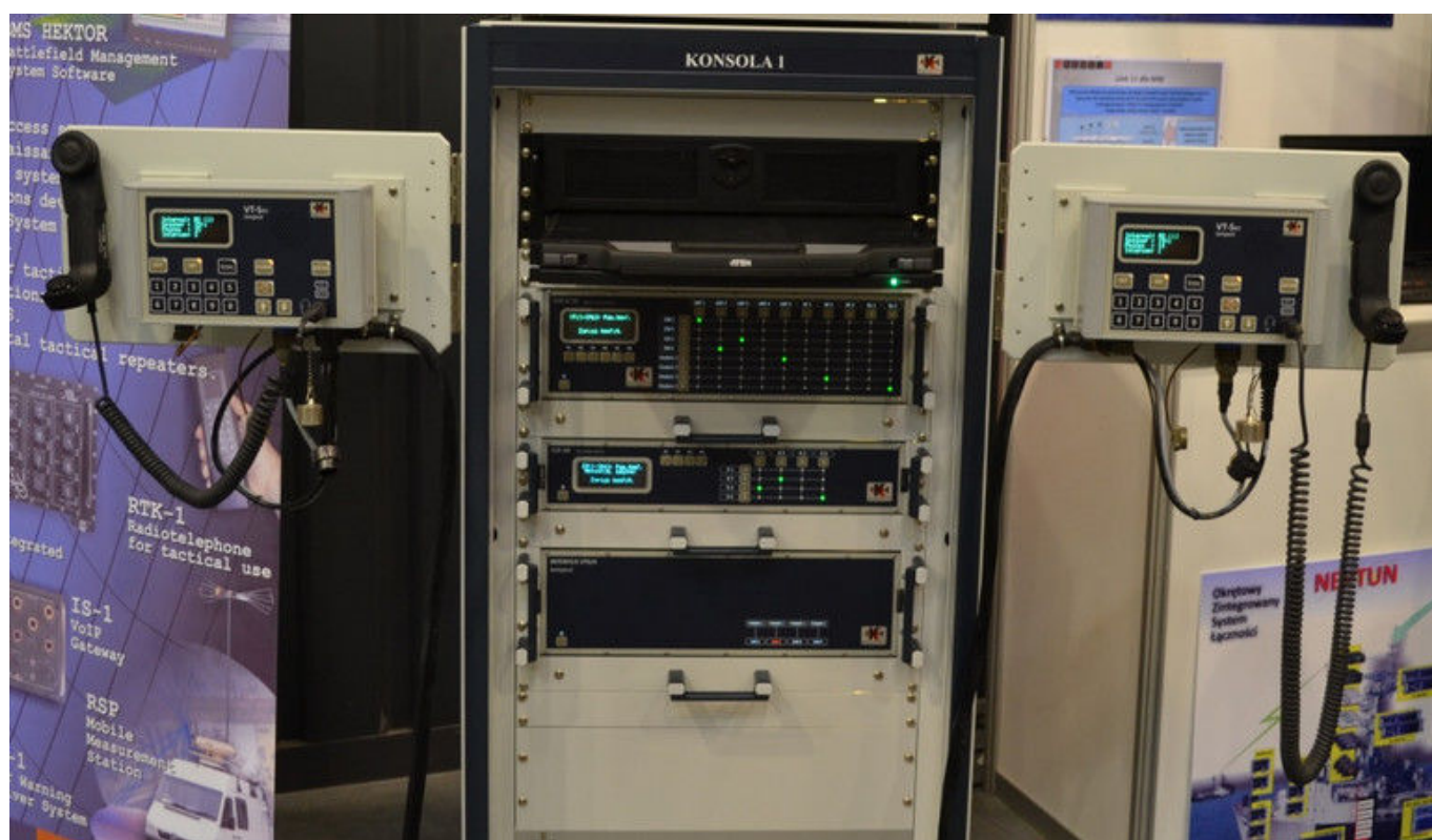
One of the mounting cabinets of the ZSŁ NEPTUN system, with the following elements installed, from the top: configuration management system (provided by the ATEN company), KenBIT KSR 8x10 Commutator, KenBIT 4x4 Commutator, and KenBIT VTS/4 interface, and two KenBIT VT-Sec terminals. Image Credit: M. Dura
