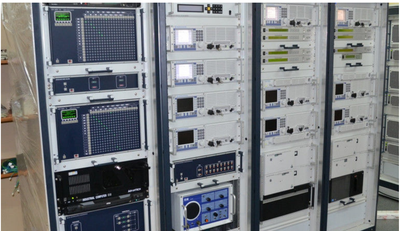
Mounting cabinets for the integrated communications suite, with embedded elements, including: KSR 16x20
